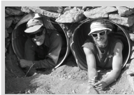
Bill Thomas (left) and Daniel Skaggs worked on a BMWF volunteer project and replaced failing culverts on Bruce Creek on the east side of The Bob, 2006.
